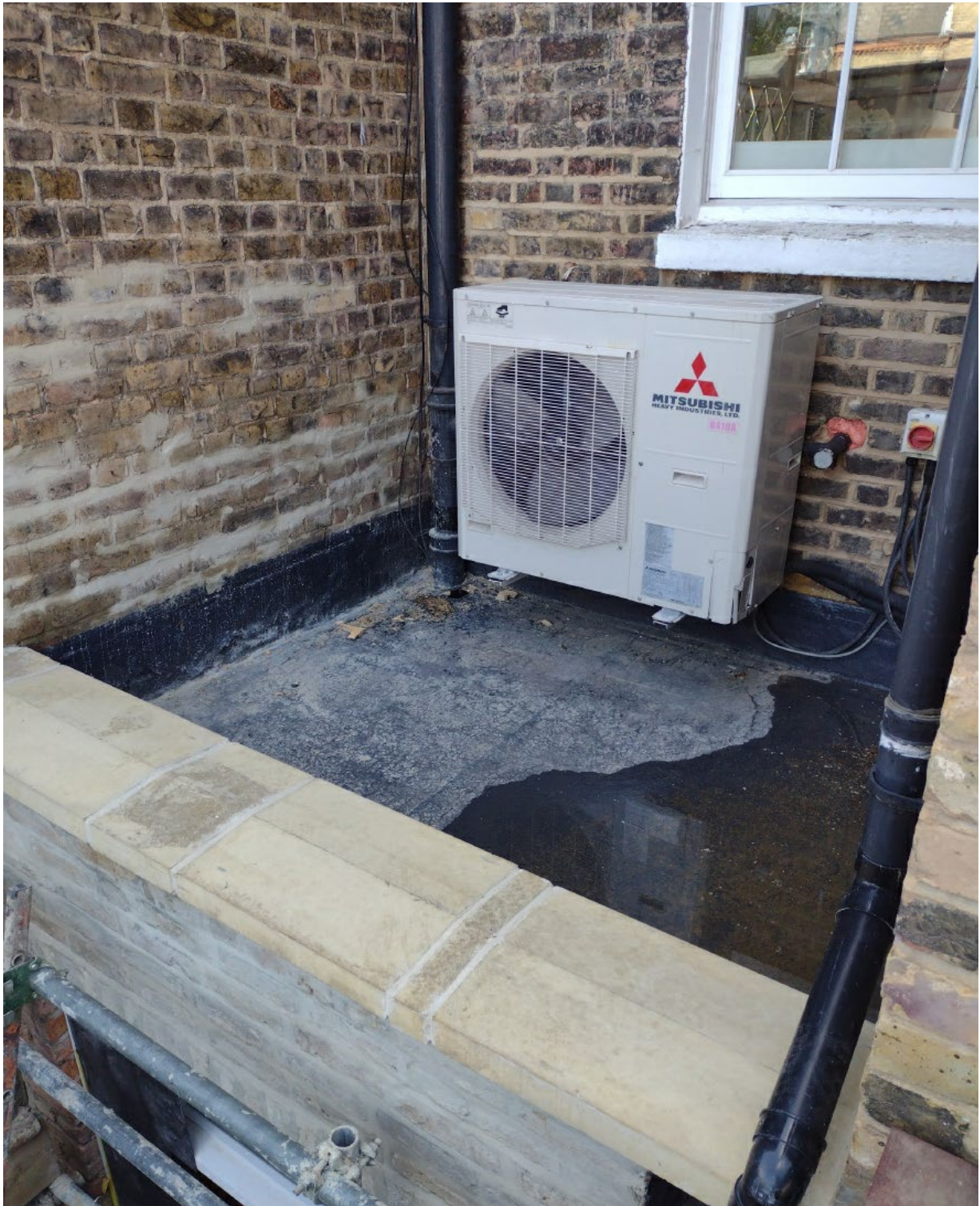
Photograph showing unauthorised unit (which has since been removed)
